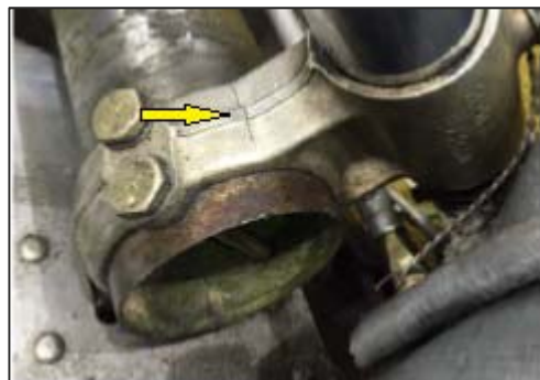
Figure 2. Crack Example (the crack is near the tip of the arrowhead)
